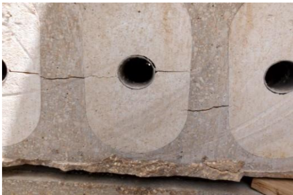
(a) Horizontal crack in webs.
