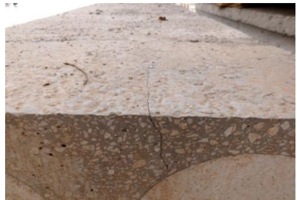
(b) Longitudinal crack in top flange.
