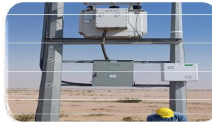
Fig. 12. Feeder Monitoring Panel
