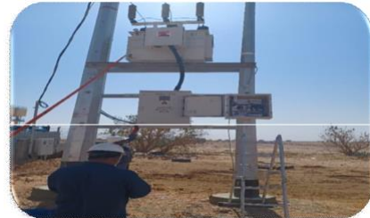
Fig. 11. Feeder Monitoring Panel installed @ the L.V. side of Distribution Transformer
