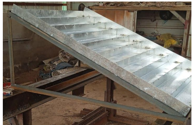
(b) Assembly of the main base with the basin of the S.S.D.U.
